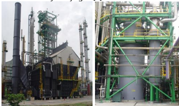
Gambar 1. Primary Reformer dan Secondary Reformer
