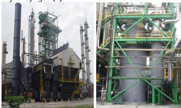
Gambar 1. Primary Reformer dan Secondary Reformer
