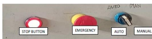
Gambar 7: Switch Stop, Emergency, auto atau manual
