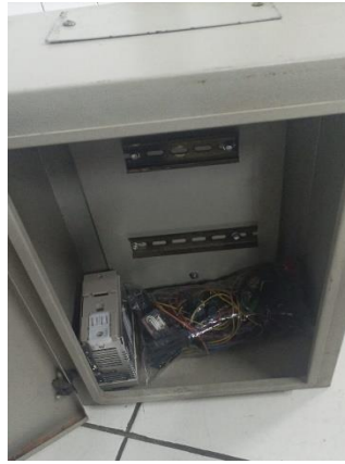
Gambar 9: Box rangkaian heater automatic run
