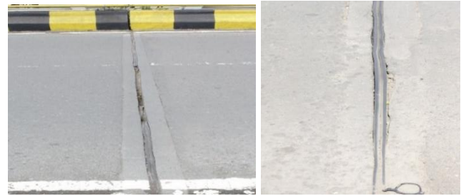
Figure 4. Damage 804. Loose of rubber adhesion. Element 4.603
