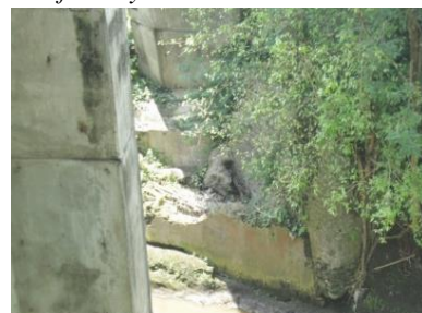
Figure 5. Rupture Damage or partial loss of the concrete
