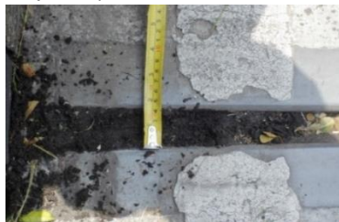
Figure 2. Damage Loose pieces in expansion joints. Element 3,600
