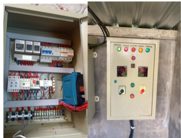
Gambar 4 Instalasi Kontrol Panel Analog
