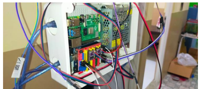
Figure 9. Panel Box Left Side View
